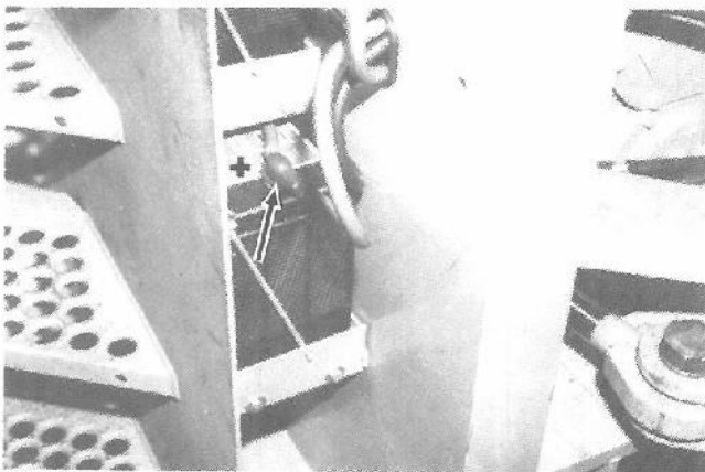
Figure 18A: Lower Battery Set Positive Terminal
